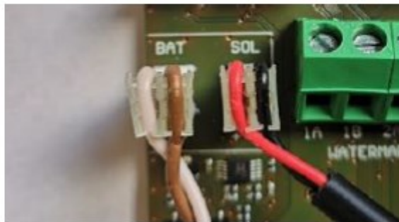
Picture 13 – Left: Battery cable, right: solar panel cable
